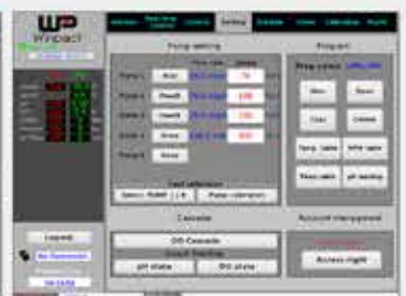
Adjustable pump setting and Cascade control
